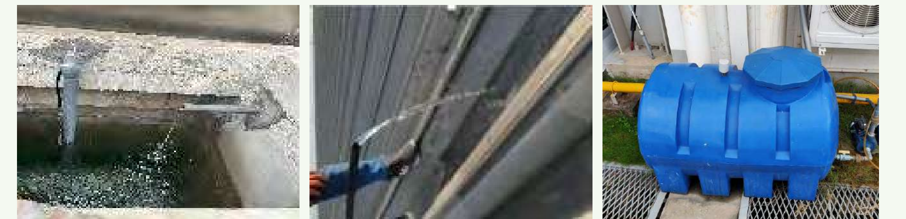
Left Image - Discharge water from drinking fountains, air compressors, rain, and glass washers converge into a 50-ton water tank / Center Image - Roof cooling in summer / Right Image - Air conditioning discharge water recycling device at the Vietnam Factory
